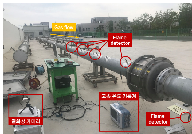
Fig. 3. Installation of high-speed temperature recorder and thermal imaging camera
